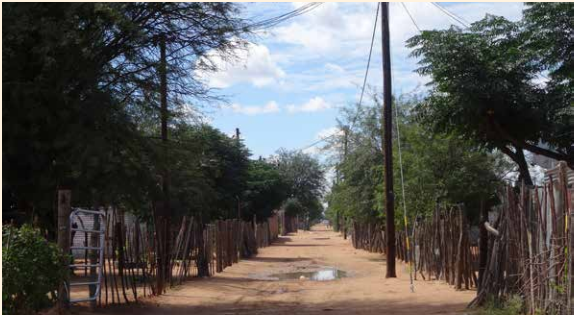
Many houses in Kanaan are connected to its electricity grid that supplies the settlement.
